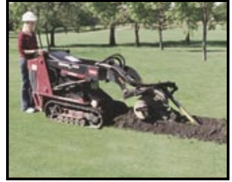
Begin trenching at the lowest point and proceed up grade. Always check with local utilities before digging.
